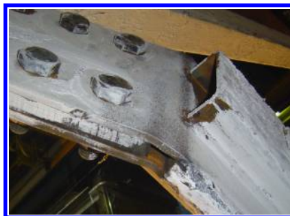
Figure 10. Deformation of double splicing plates at plastic hinge node 3 or 7.
