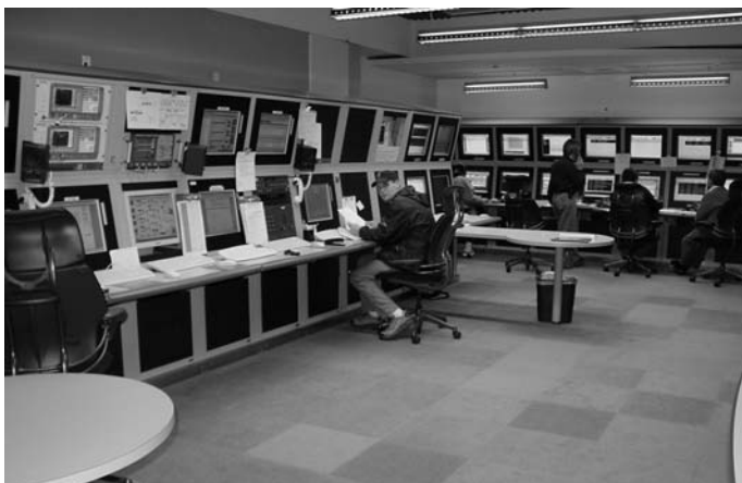
Figure 7.20 XM operations control center.
